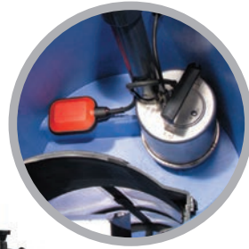
Continuous pumper unit
